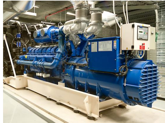
DRUPS Generator & MS Rooms
